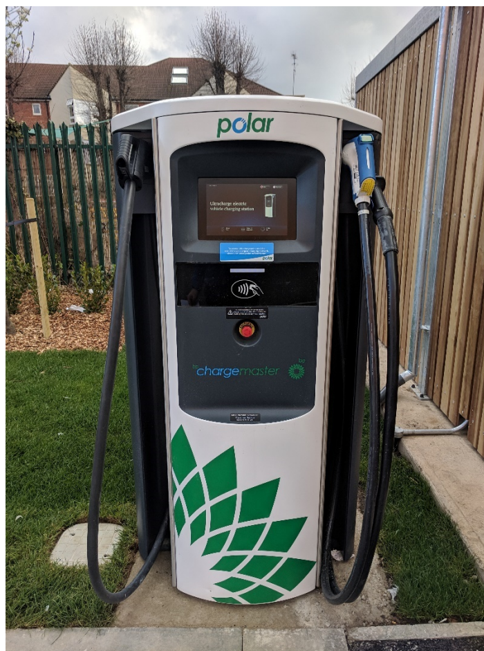
Rapid Charger at the Council's new leisure centre on Farnham Road in 2019 – Charges Electric Car in 30 minutes. The Council is looking to expand its rapid charger network to 10 rapid chargers by the end of 2021.
